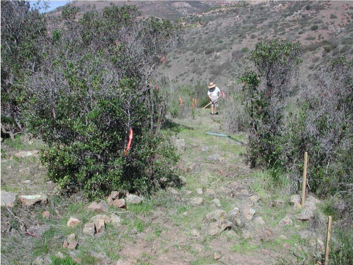
Del Dios Gorge Trail during the “clearing and grubbing” stage of construction.
