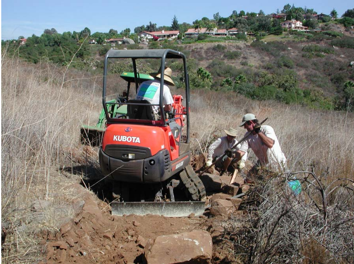
Senior Ranger Dave Hekel struggles to get the mini-excavator back on track.
